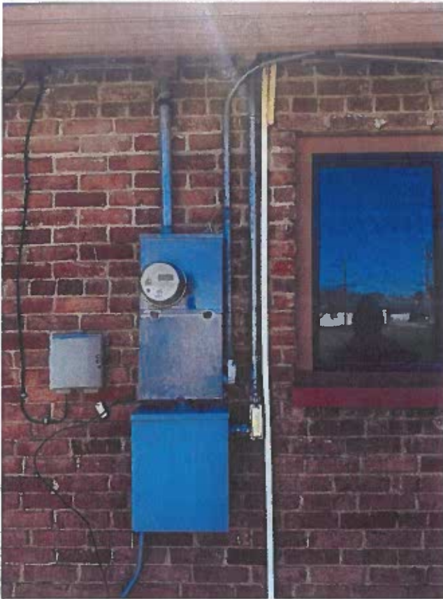
Electrical Panel Not for Commercial Use
