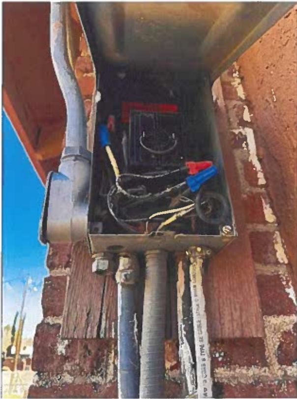
Electrical Box Not up to Code for Commercial Use
