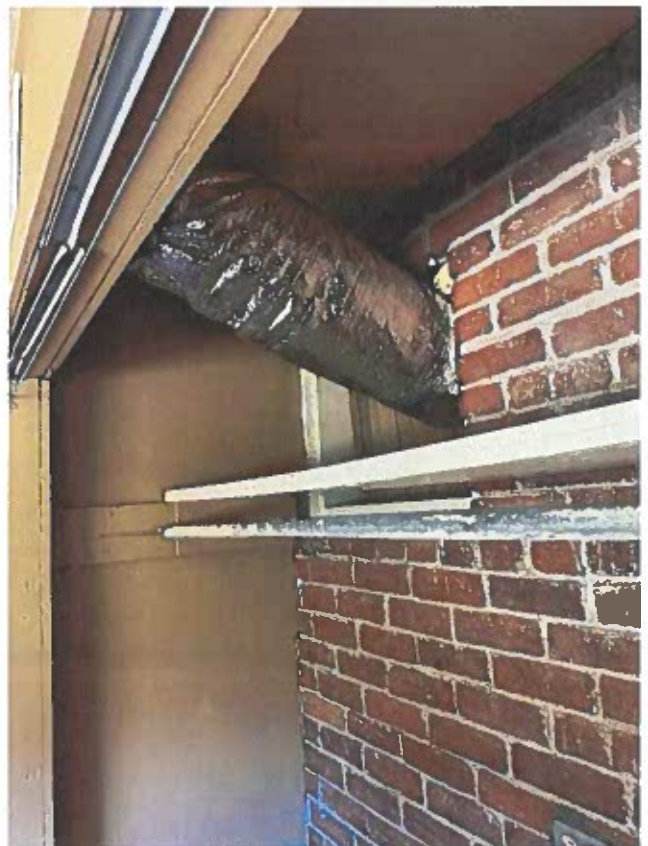
HVAC Not up to Code for Commercial Use
