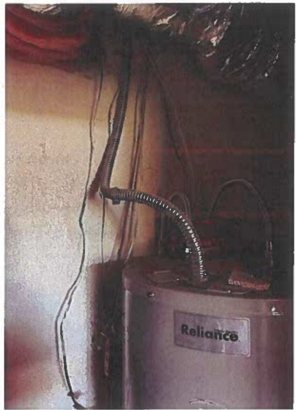
- Water Heater Needs to be Brought up to Code
