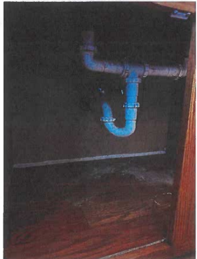
- P Trap Missing, Sink has Leak, Not up to Code
