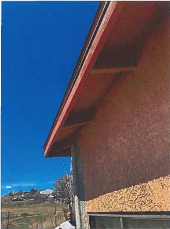
- Trusses Rotted Under Eaves
