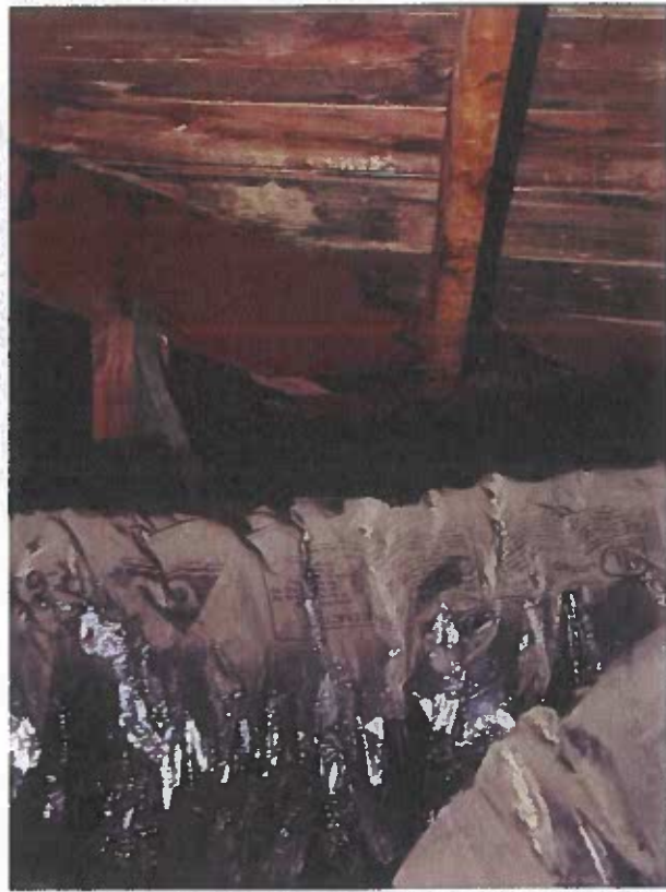
Broken Trusses in Attic
