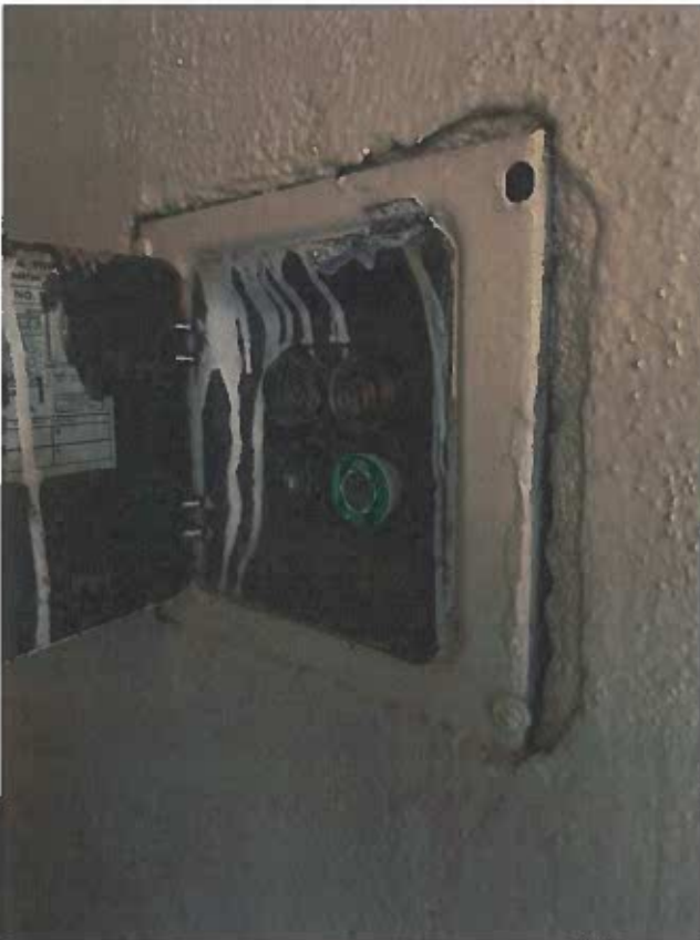
Electrical Not up to Commercial Code
