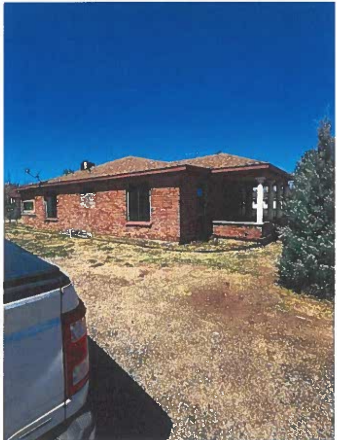
Foundation shows signs of deterioration.
