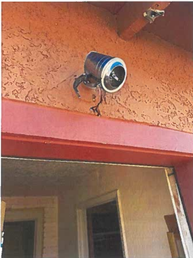
Item needs to be removed from Light Fixture and Brought to Code
