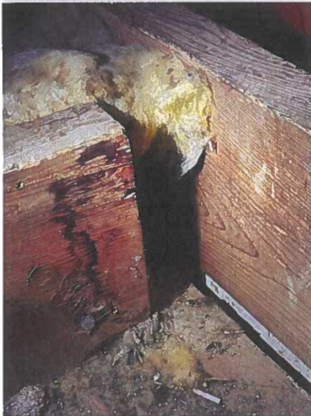
Ceiling Joist Cut Too Short
