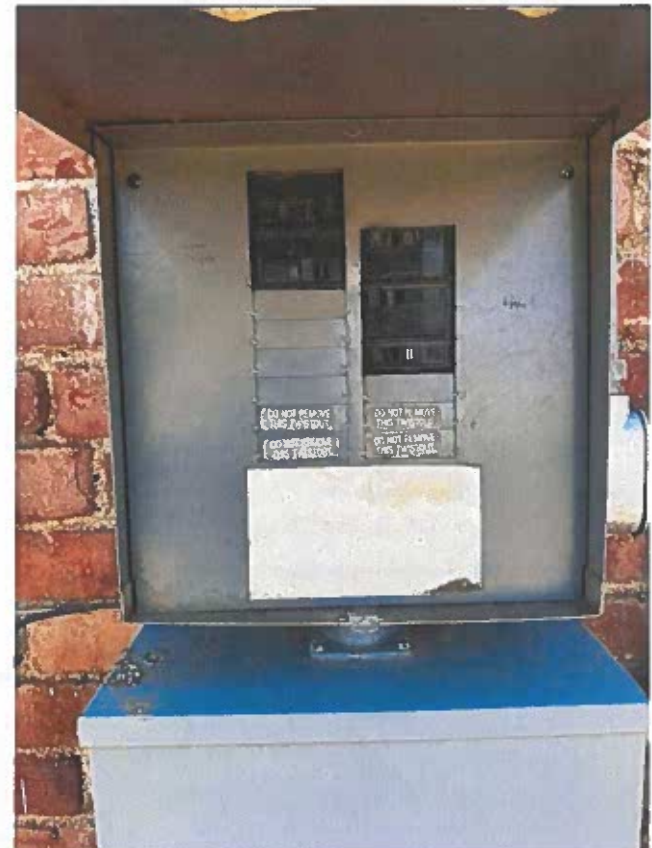
Electrical Panel Needs to be Upgraded
