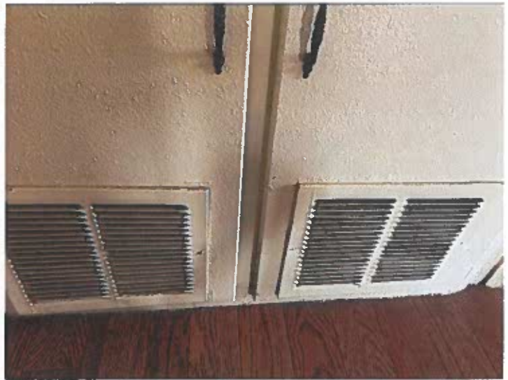
HVAC Fresh Air Return – Needs to be Brought up to Code
