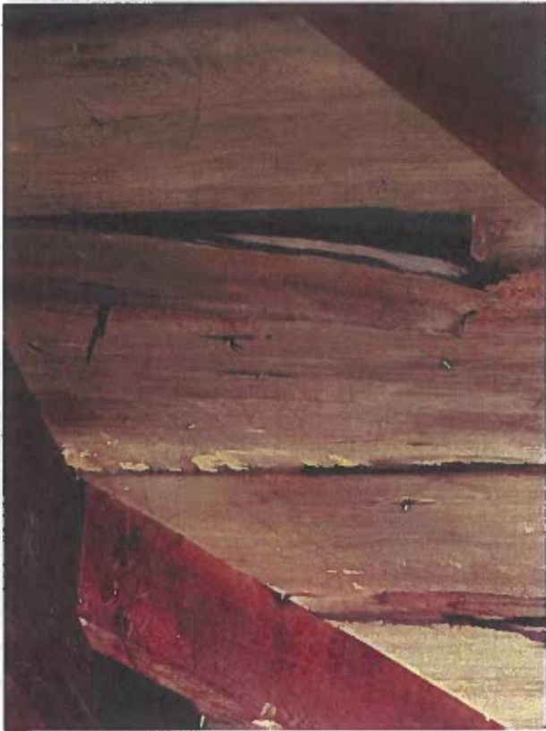
Broken Truss in Attic
