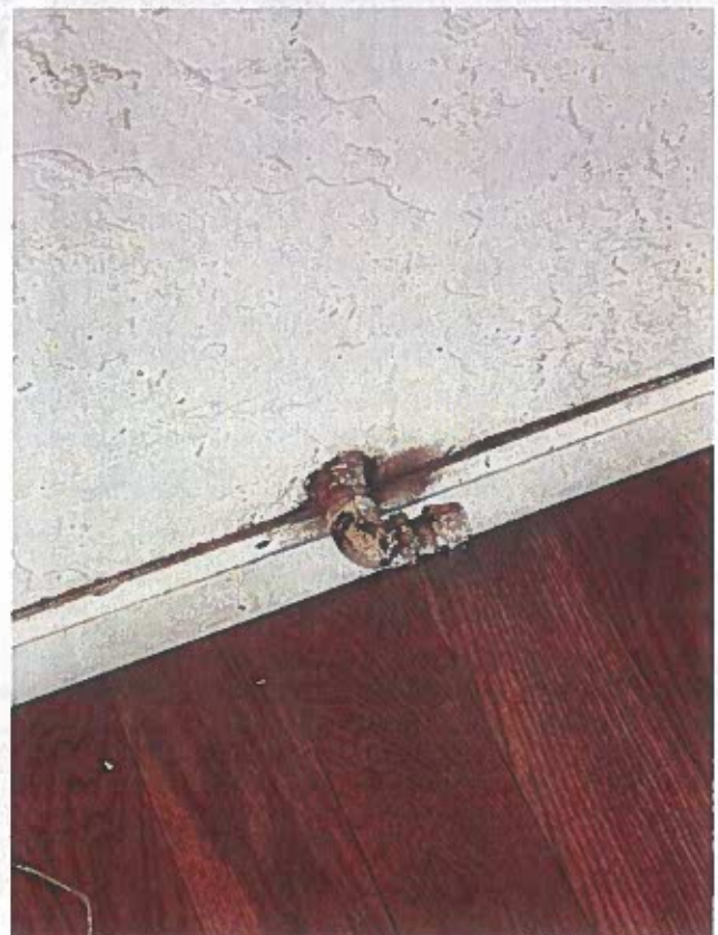
Gas Pipe – Unknown Origin
