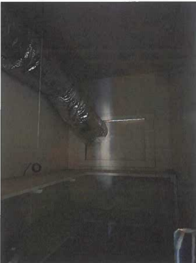
HVAC Ducting Not Up to Residential or Commercial Code
