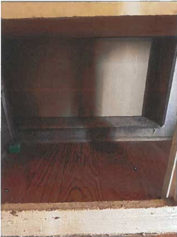
HVAC Abandoned Fresh Air Vent Abandoned
