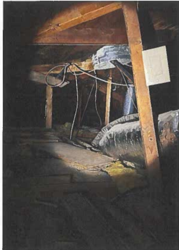
Electrical in Attic Not to Code
